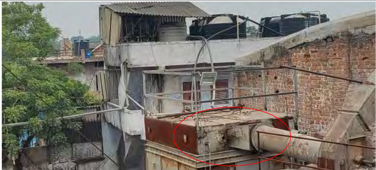
Holes was found at top portion of Bag Filter due to corrosion
