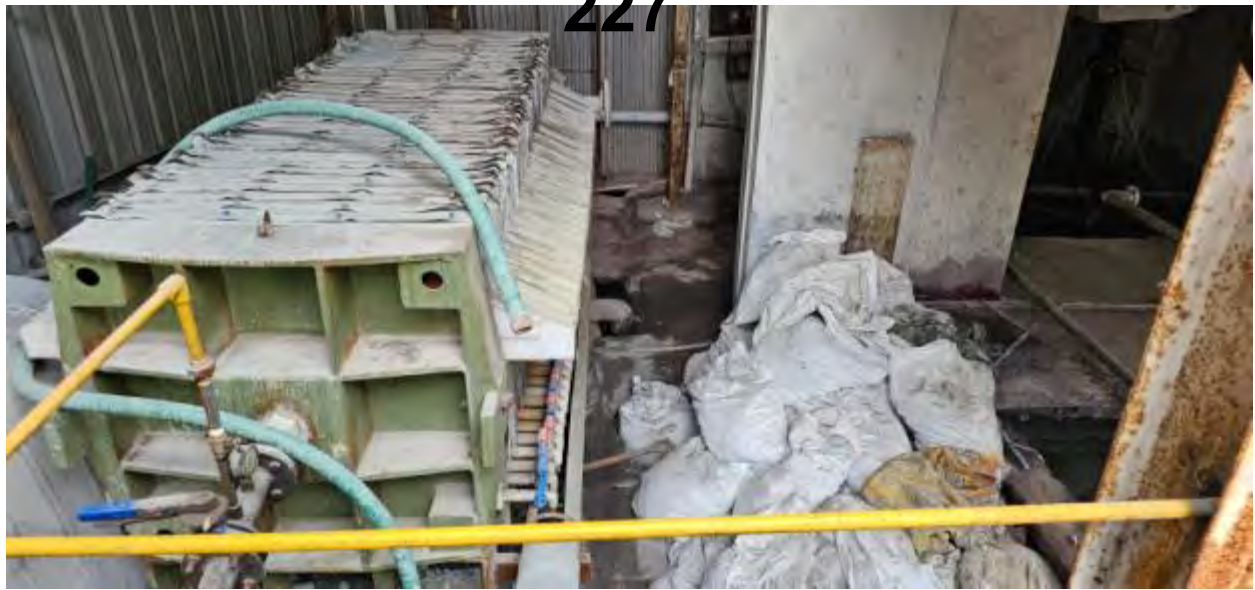
Filter Press & ETP Sludge
