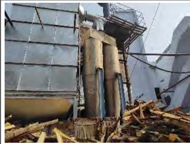
Bag filter + Multi cyclone
